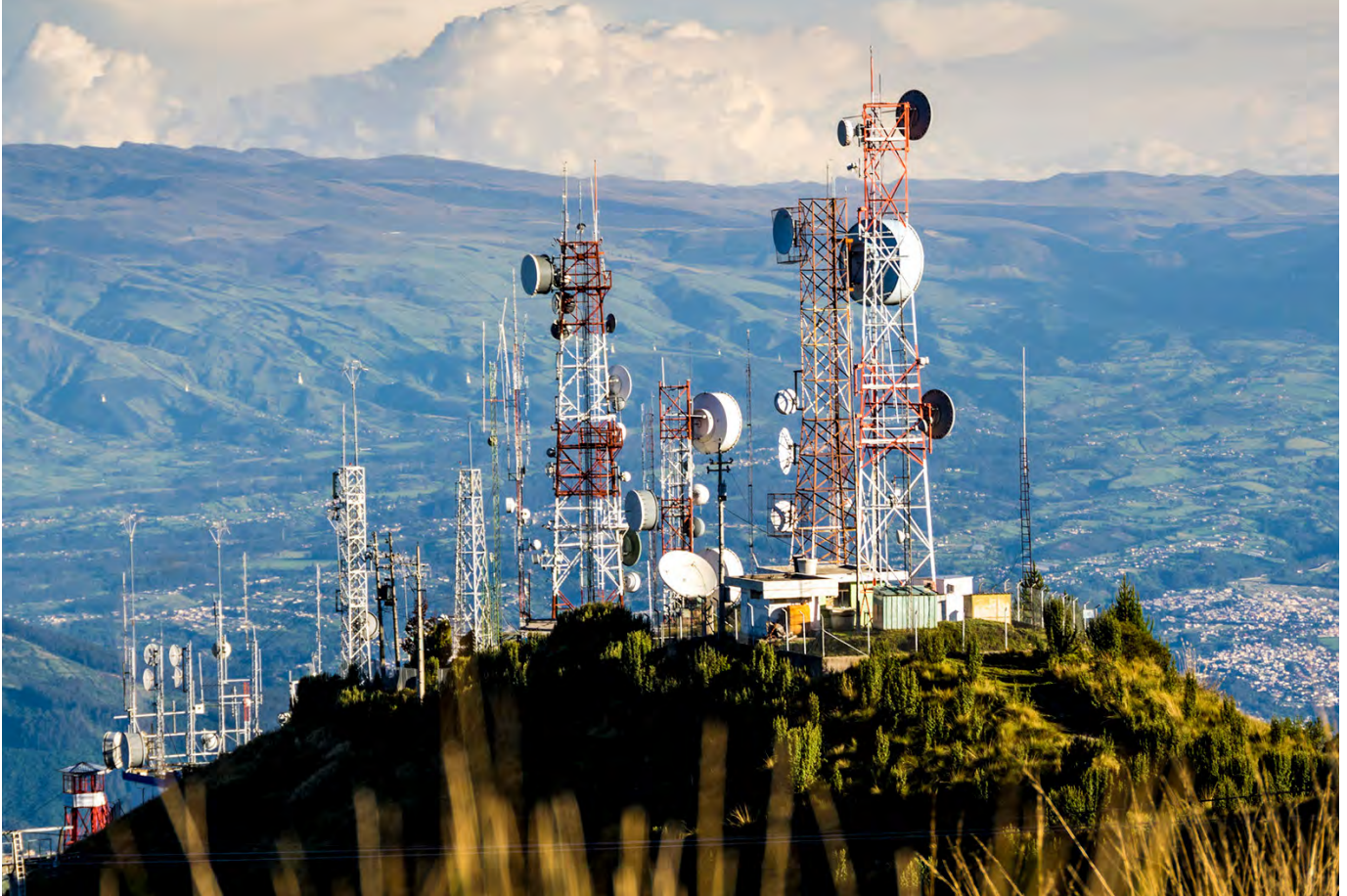
Cellular, TV, and radio antennas are arrayed along a mountaintop near Quito, Ecuador, with the slopes of the Cotopaxi volcano visible in the background. (Photo by Michael Müller/iStock)
