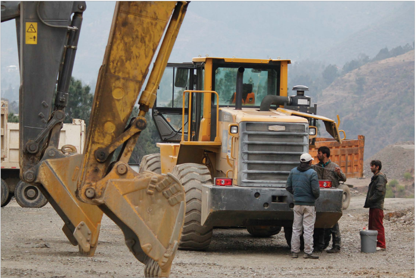
Construction workers work on the Havelian-Thakot section of the Hazara Motorway, a major project of the China-Pakistan Economic Corridor, in the Salhad area of Abbottabad, Pakistan, on January 29, 2017. (Photo by Sultan Dogar/iStock)
